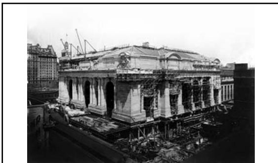
Above: May 1912. Scaffolding still surrounds the building as construction continues. The photograph was taken from a building on the south-side of 42nd Street. The east-side (Depew Place) facade (at right) as well as the south/main (42nd Street) facade (at left) are in view.
