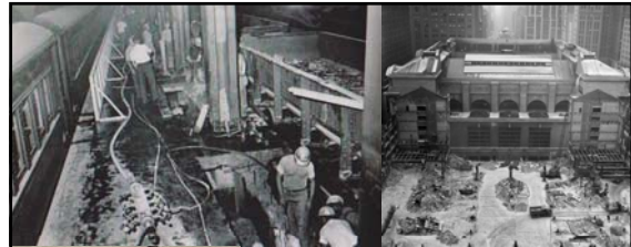
Left T&B: support for the 45K-ton steel frame utilized two-hundred existing columns plus an additional ninety-five sunk into bedrock fifty-five feet below Park Avenue for what became the Pan Am Building Right: the long hidden back facade of GCT exposed when the Grand Central Terminal Office Building was demolished for the construction of the new 59-story Pan Am Building (January 1961)
