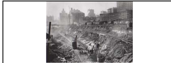
“One of the features that render the construction of the new Grand Central terminal station a work of unprecedented and monumental proportions, is the vast amount of preliminary excavation that has to be carried out before a single track of the station yard, or a single brick or stone of the station building can be laid. This excavation amounts to a total of over 2,000,000 cubic yards, a large part of which is rock. The blasting out and digging of this material in the heart of a great city, and its removal and disposal many miles from the point of excavation, is in itself a task of huge proportions.” Scientific American, September 16 th 1905 Above: view looking south (from 49 th Street) of train yard excavation 14
